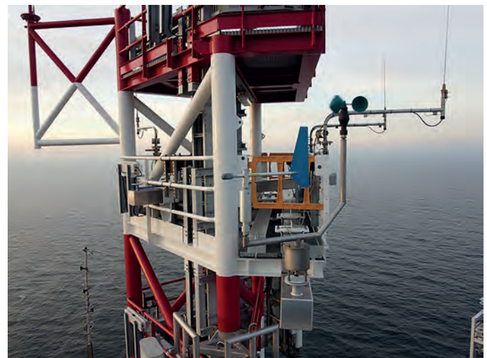
▲ Figure 2: anemometer, windvane and other instruments attached to a tower on a wind farm platform, source: KNMI
