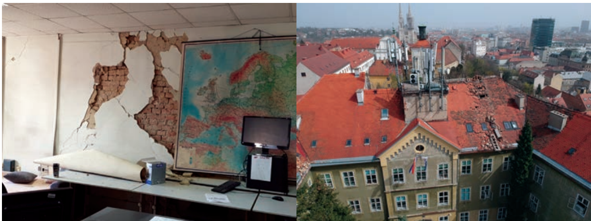
▲ Figure 1. Headquarters of Croatian Meteorological and Hydrological Services after the earthquake (source: DHMZ)
